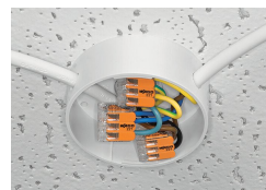
Lighting distribution in a ceiling canopy
